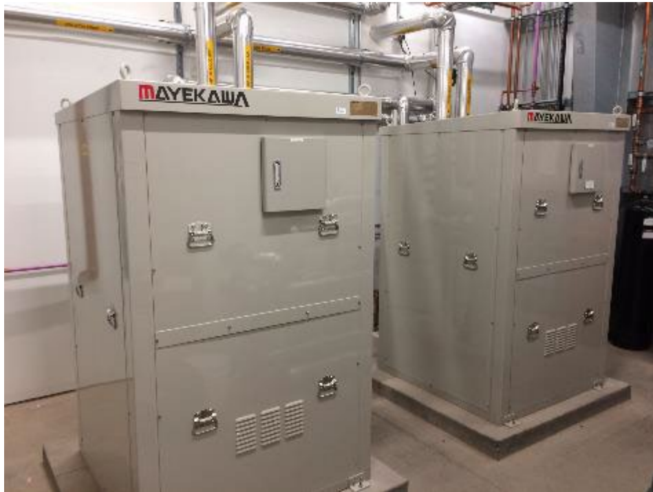
(2) UNIMO ww units installed in Mechanical Room
