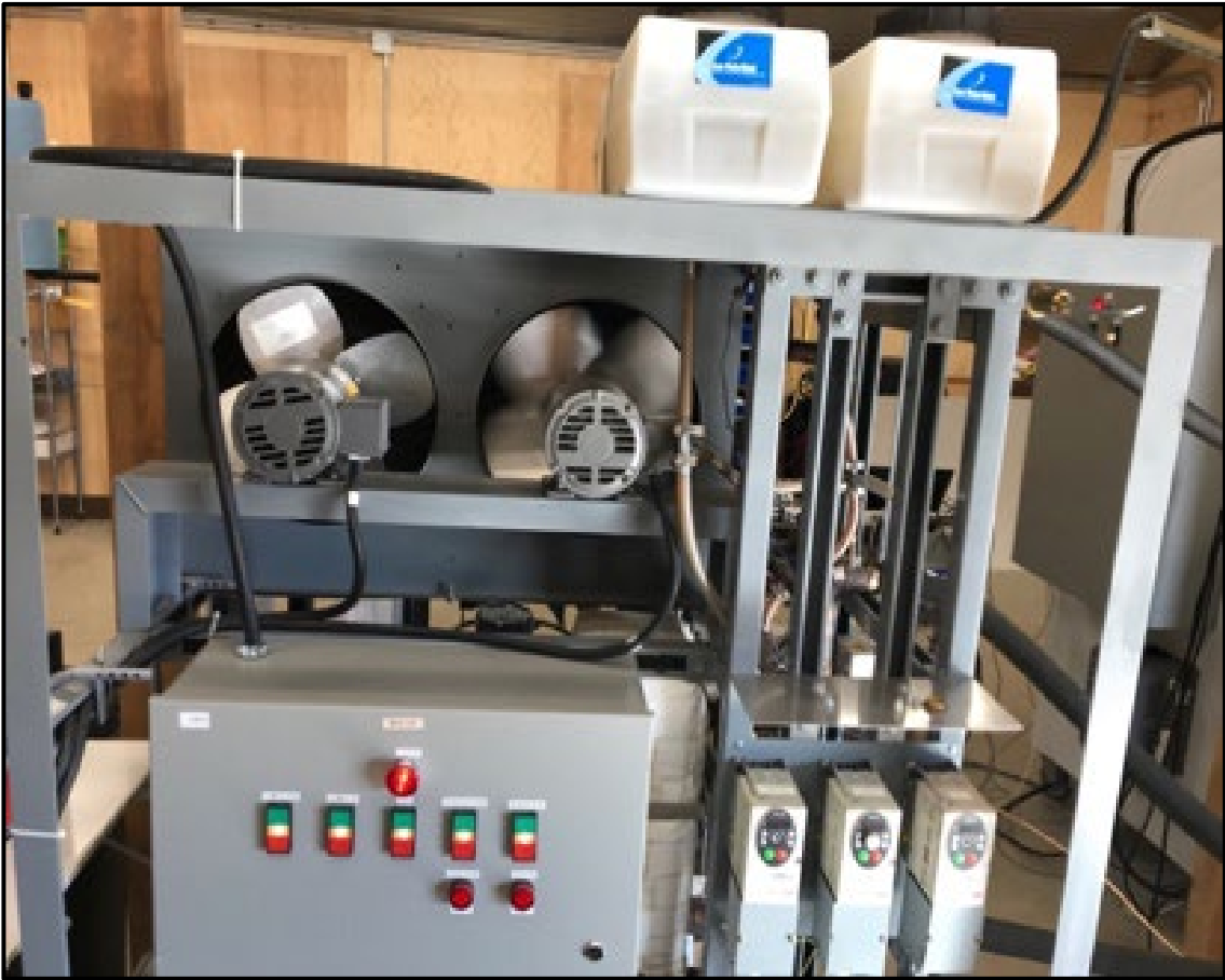
Prototype Showing Controllers and ASDs
